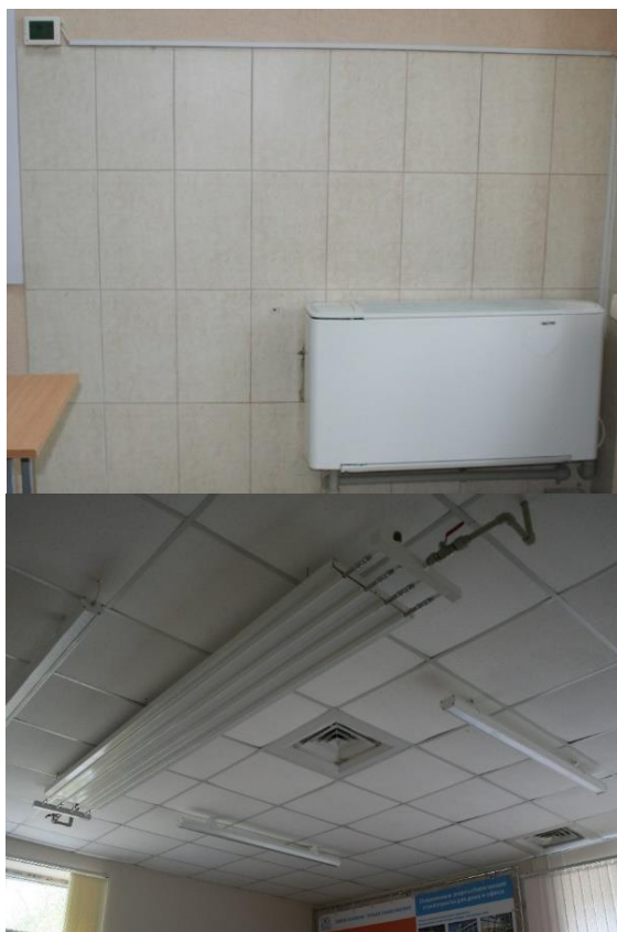
Figure 2 – Wall-mounted Vita fan coil with a capacity of 5 kW with a software control unit (left) and a climatic radiation panel produced by Effi
