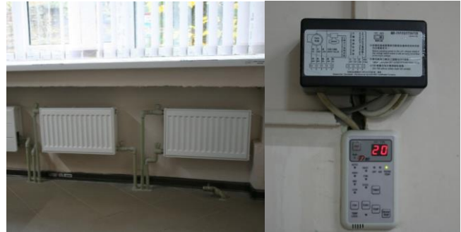
Figure 3 – Jaga wall-mounted convector and two steel wall-mounted Korado radiators (from left to right) and a programmable remote control for intermittent electric underfloor heating from Teplolux with a capacity of 3 kW in one of the classrooms
