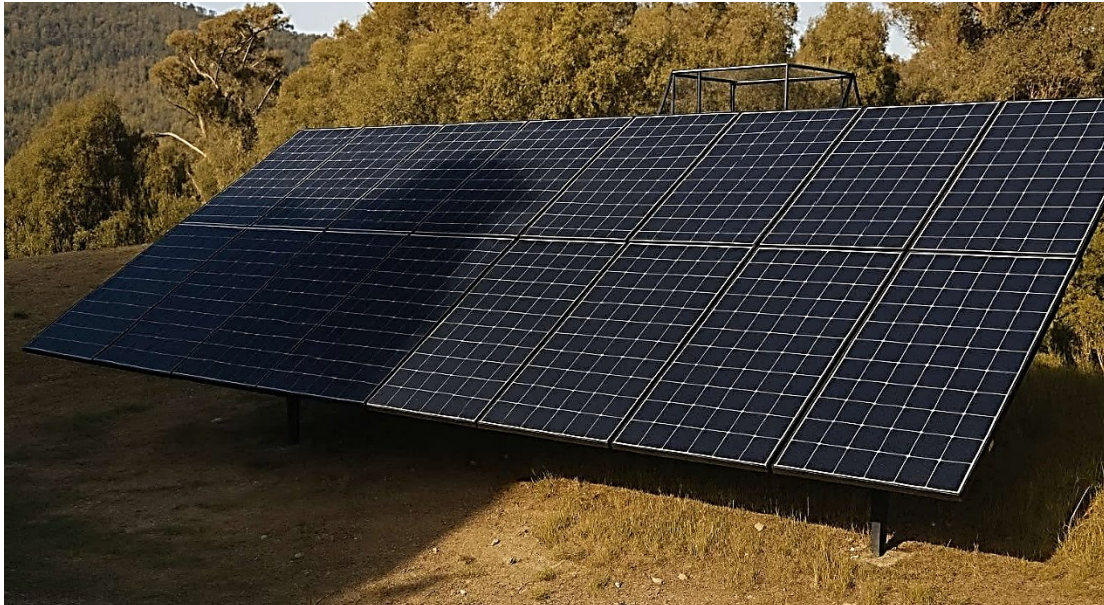
Fig. 1. Example of shading of photovoltaic panels affecting system performance.
