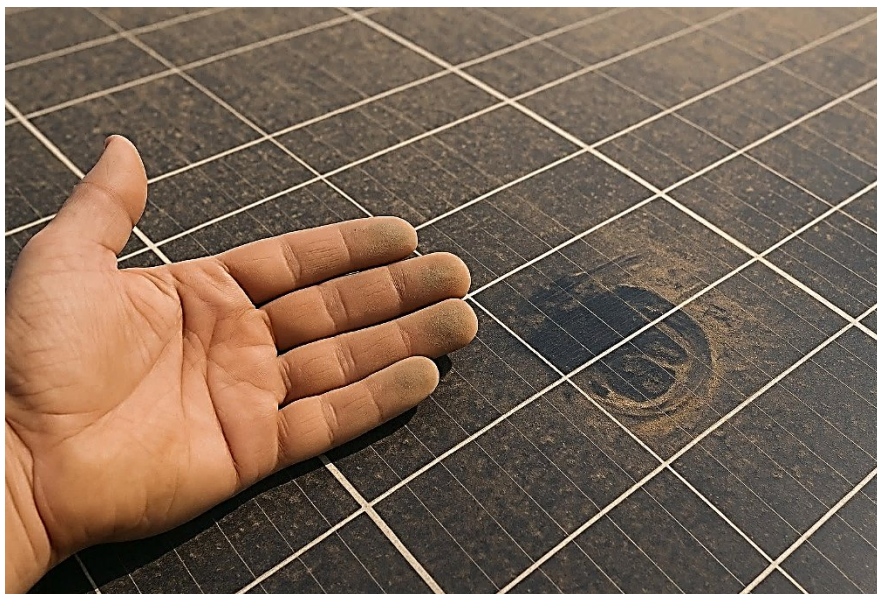
Fig. 2. Example of dust contamination of photovoltaic panels affecting system performance.
